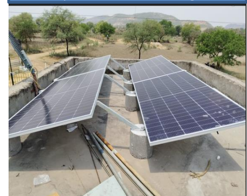
FY 24-25 ,2 KW Grid Roof solar -4 no system installed at LC gates
