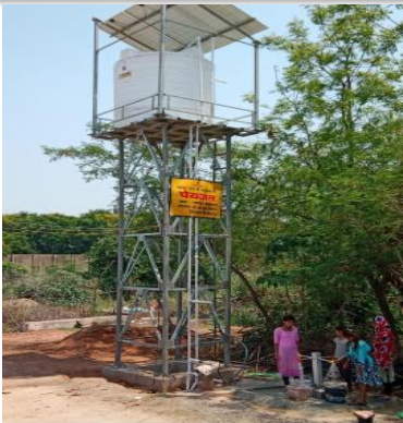
OFFSITE: Solar Pump
