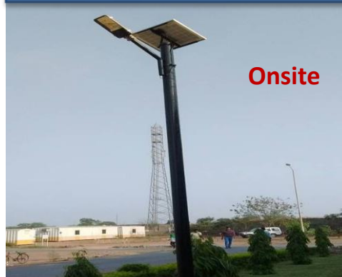
PV Solar Street Light Inside Plant
